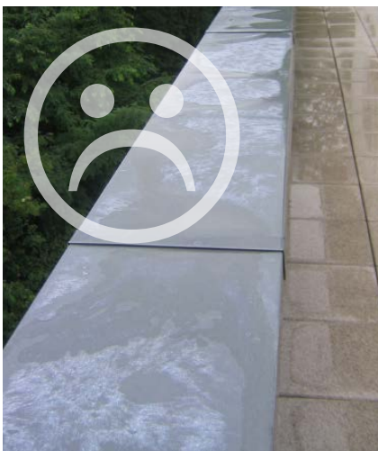
Zinc hydroxide formation due to insufficient slope
